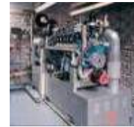
Heat recovery (CHP)
